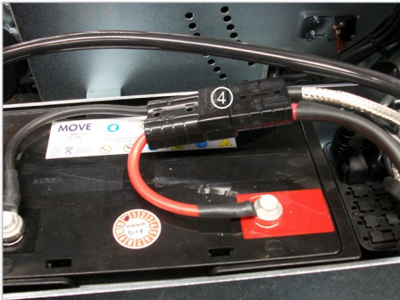
Fig. 52: Main Cable battery
