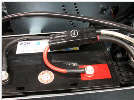
Fig. 47: Main Cable battery
