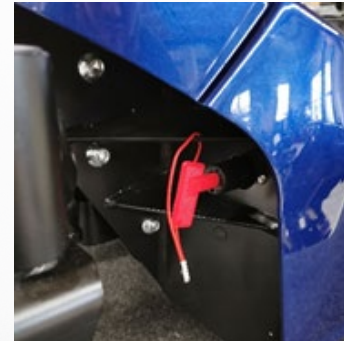
Fig. 110: Battery dicon. switch, inactive
