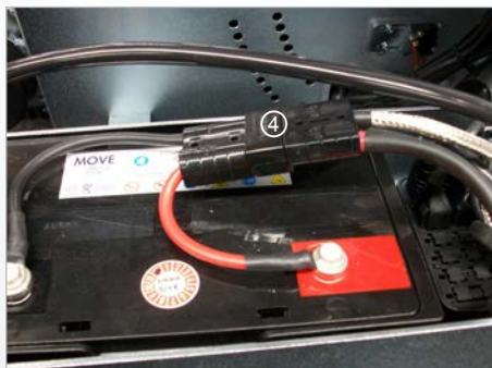
Fig. 53: Main Cable battery
